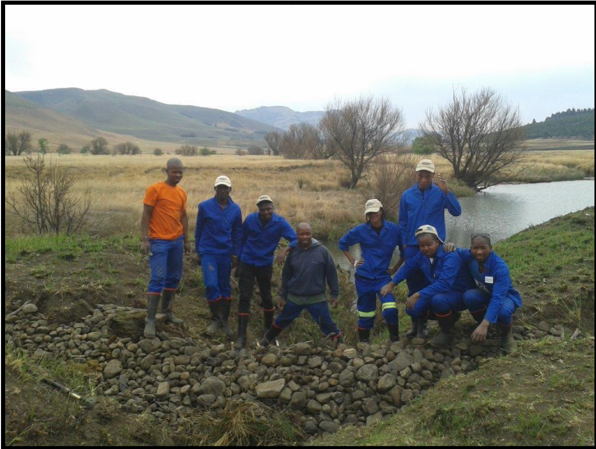
Above – Rehabilitation of a trench in a wetland by the EWT EcoRangers - Tusa Farm Underberg
