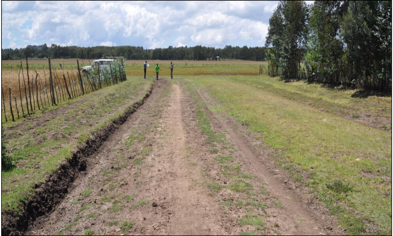
Figure 2: A recently graded road ending on the lake boundary. PHOTO courtesy of EAWLS. 25/10/2016
