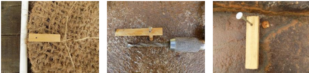
Figure 19. Left: Plug, nail and washer; Middle: brace and masonry bit; Right: pine washer, galvanised pin and dowel plug inserted after hand drilling
