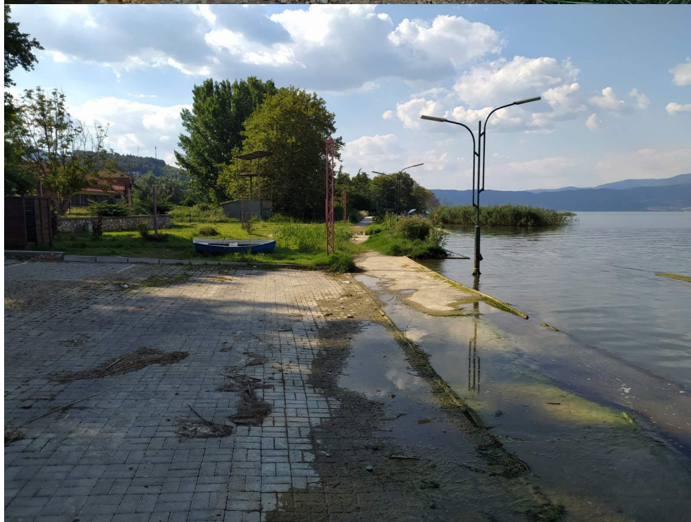
Figure 1 Photos of damaged and flooded coastal walking path. (Courtesy of M. Velchev; 22.07.2020)
