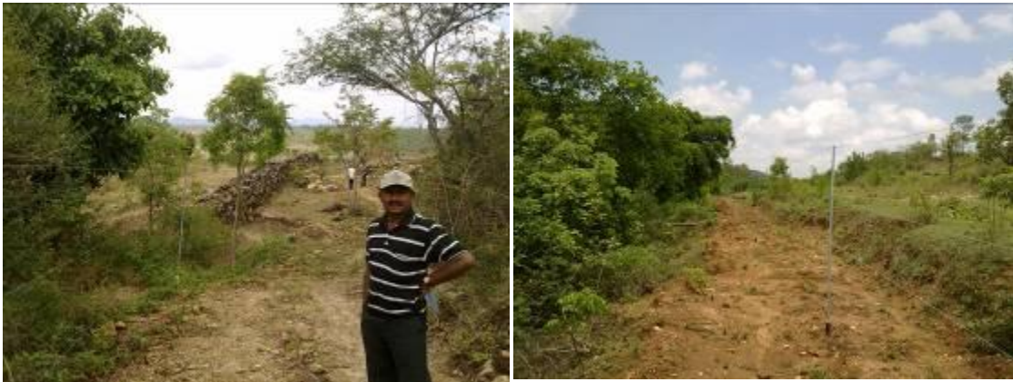
Fig. 9 Rubbel wall with AC charged fencing in the Bilaganaguppa village (left) and AC charged fencing in the Bilaganaguppa Village (right)
