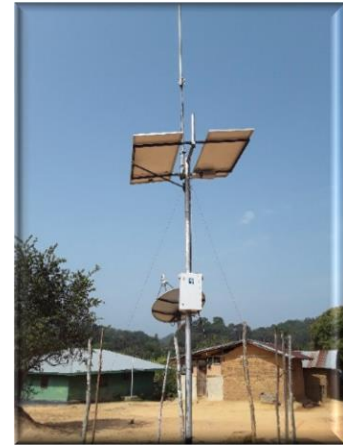
Figure 2: Solar Mast in Camp Alpha
